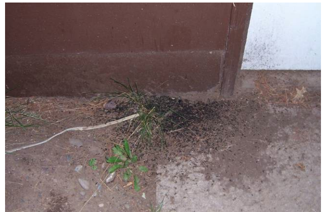
Bat guano in front of garage
