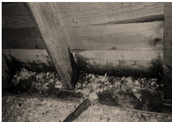
Figure 6. Urine and feces below an attic vent where flying squirrels were exiting the home. Photo by S. Vantassel.
