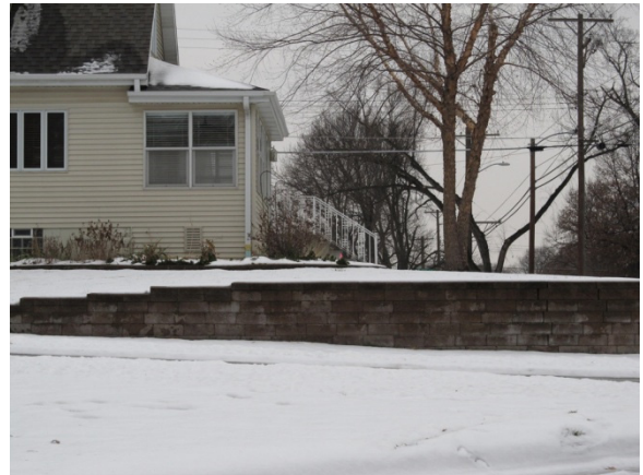
Figure 2. Falls from embankments can occur if you are distracted. Photo by Stephen M. Vantassel.
