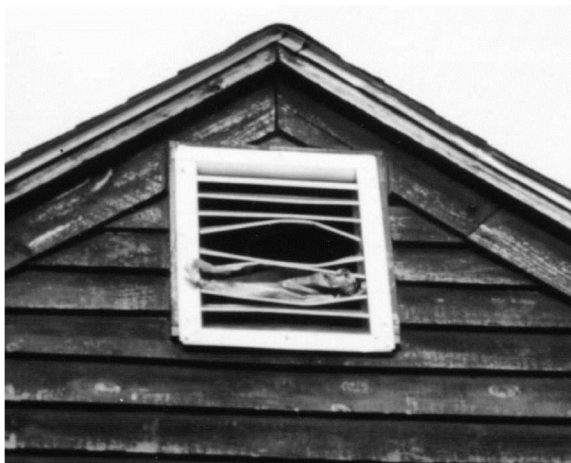
Figure 5. A raccoon entered this attic through the vent. Photo by Stephen M. Vantassel.
