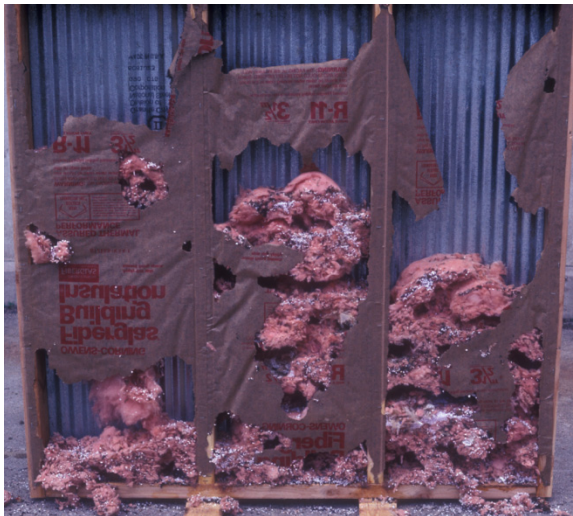
Figure 4. Insulation that has been damaged by house mice. Photo by Robert M. Timm.
