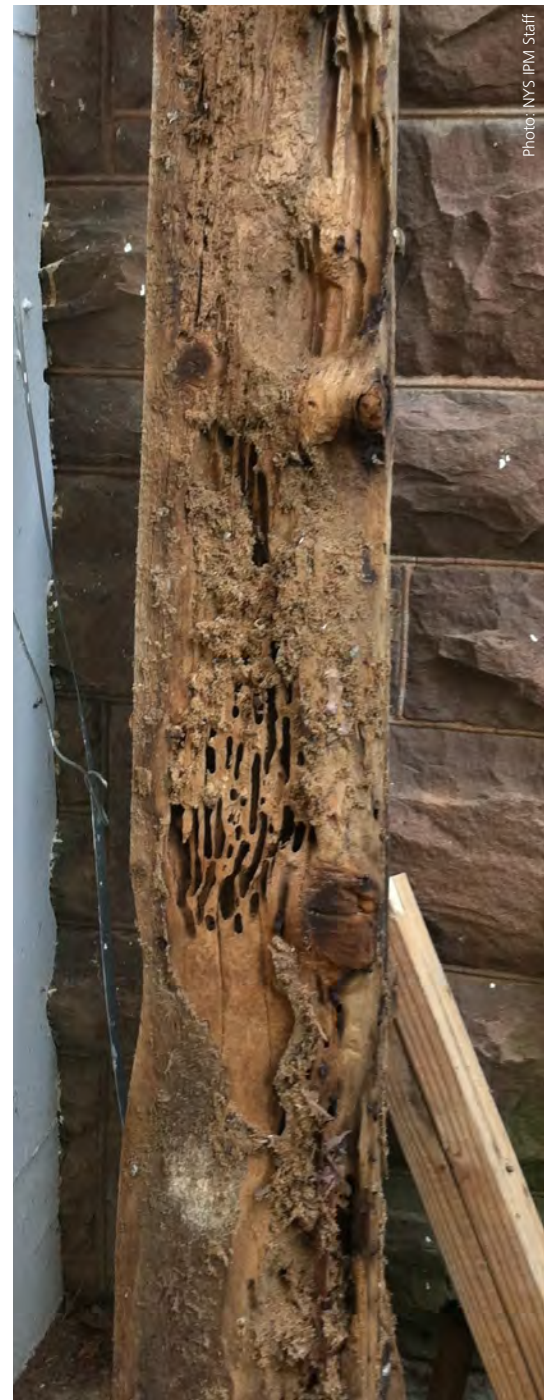
Black Carpenter Ant damage
